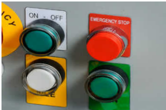
Control panel labels
