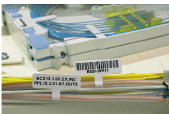
Fibre optic cable markers
