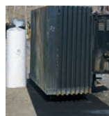
Ideal underneath leaking transformers.
