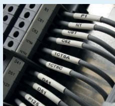
Wire & Cable Marking
