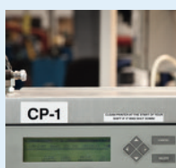
Control Panel and Electrical Panel Labels
