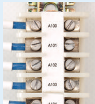
Terminal Block Marking
