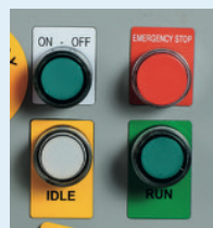
Control Panel Labelling
