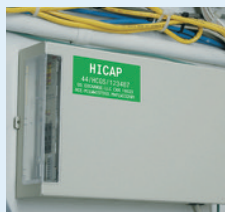
Control Panel Labelling
