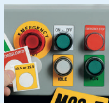
Control Panel Marking
